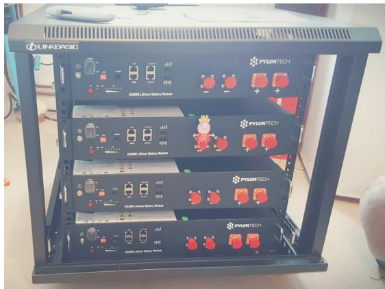
10 kWh battery storage
